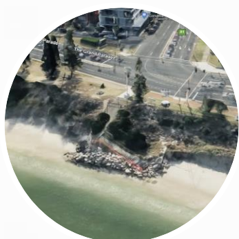
4. Damaged inaccessible stair
