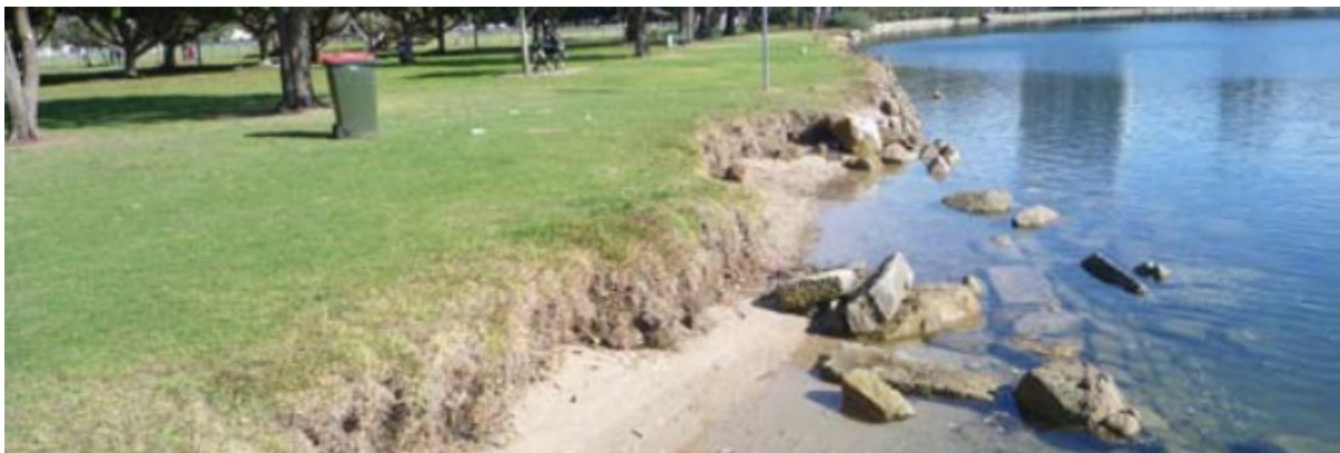
Shoreline erosion at Cahill Park
